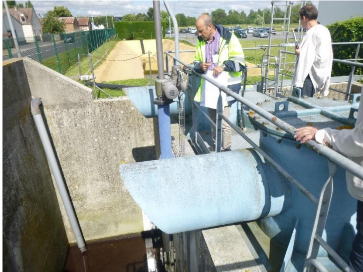
Figure 5-5 : Station de pompage de SANOFI
