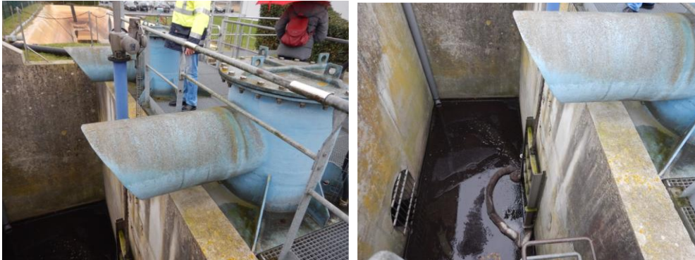
Figure 7-1 : Station de pompage de SANOFI
